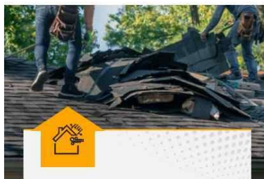
Roof Storm/Wind/Hail Repair
