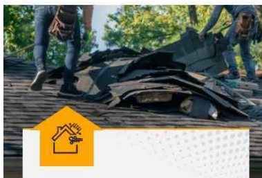
Roof Storm/Wind/Hail Repair
